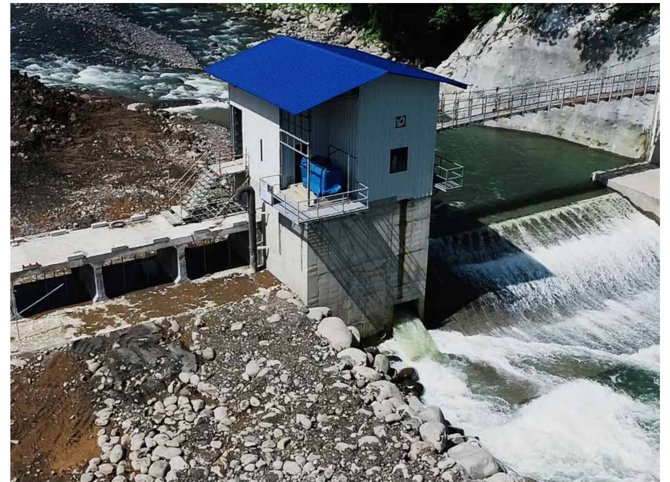
THE SHAPE OF WATER. Apo Agua has completed the construction of its run-off type intake weir across the Tamugan River, which will aid in managing the rate and volume of raw water diverted from the surface water source before it is conveyed to the water treatment plant.
